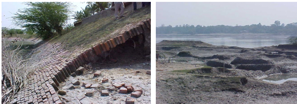
Plate 1: Distressed (a) Brick Pitched (L) and (b) Earthen Embankment (R)
